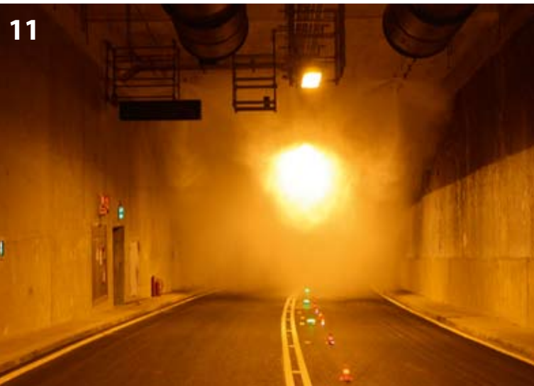
Commissioning the test of FFFS in the new Tyne Tunnel in February 2011 [8]
