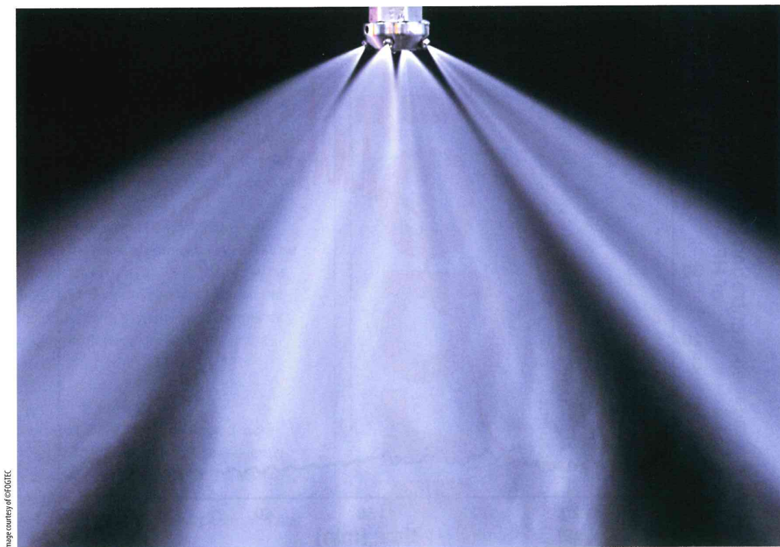
► Figure 3: Spraying high-pressure watermist nozzle.
